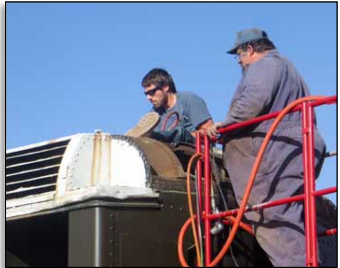
Spencer Piontkowski (L) and Robert Smith at work on the roof of coach SD&A 250 Ron Hyatt
