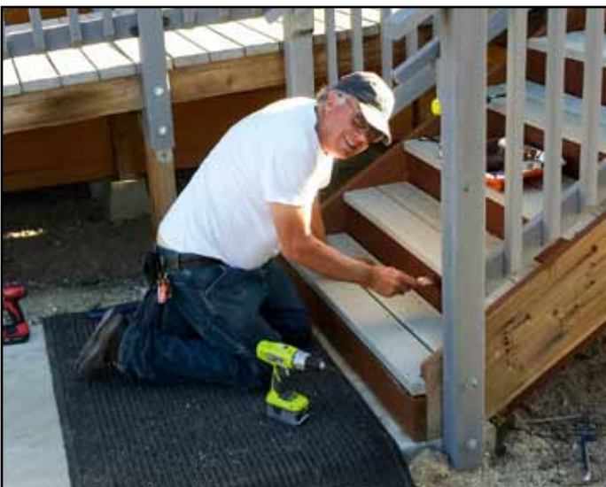
Facilities Director Frank Denison puts the finishing touches on repairs to the stairs of the Campo Depot. Jim Lundquist
